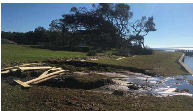
Bulkhead damage at Camp Albemarle after Hurricane Florence. This bulkhead is adjacent to the living shoreline.
