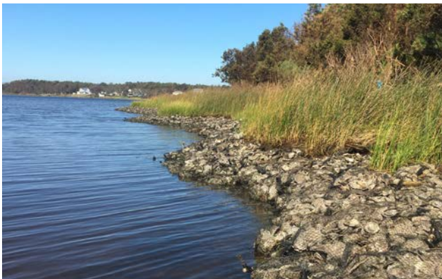
Camp Albemarle site after living shoreline installation. (Image taken a few days after Hurricane Florence)
