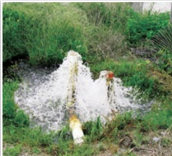
Stormwater gushes out of pipes behind a sand dune in Atlantic Beach.
