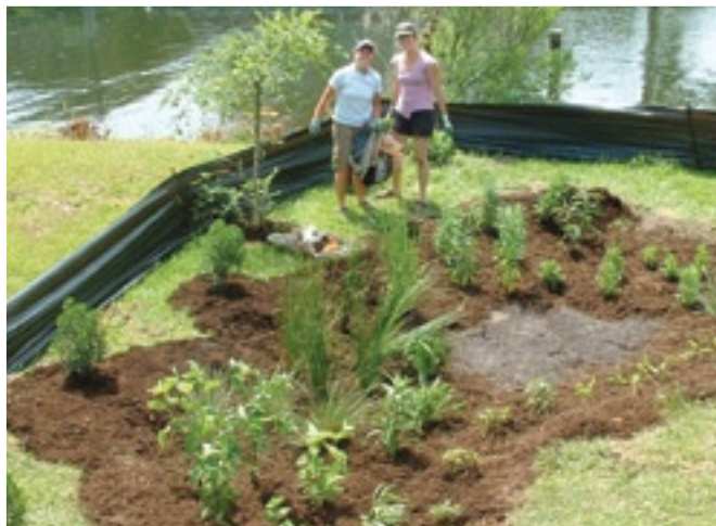
Federation staffers SARA HALLAS, left, and ERIN FLECKENSTEIN build a rain garden at the federation's new office in Manteo.
