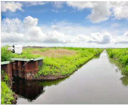
This pump redirects drainage water into the project area.
